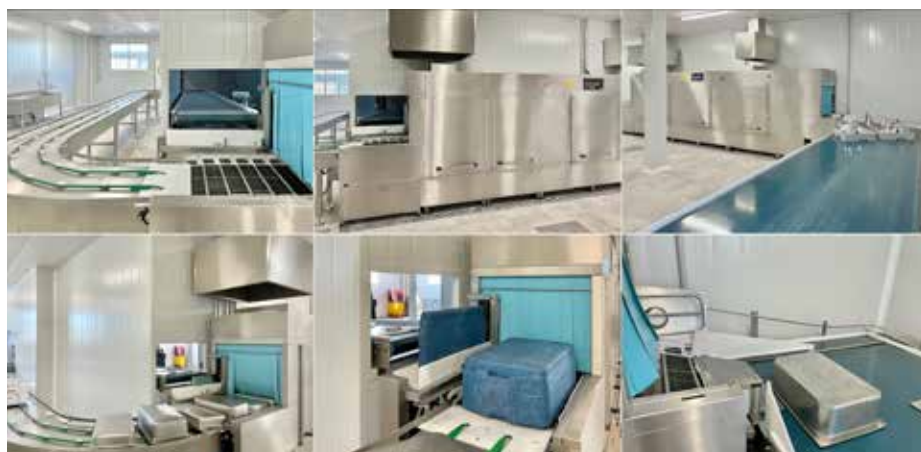
Automated washing system
